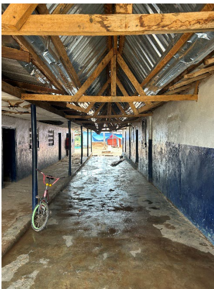
The roof over the corridor at the Dorothy Cooper Kindergarten and Primary School in Bong County, Liberia, leaks during the rain, January 8, 2026. © 2026 Human Rights Watch
