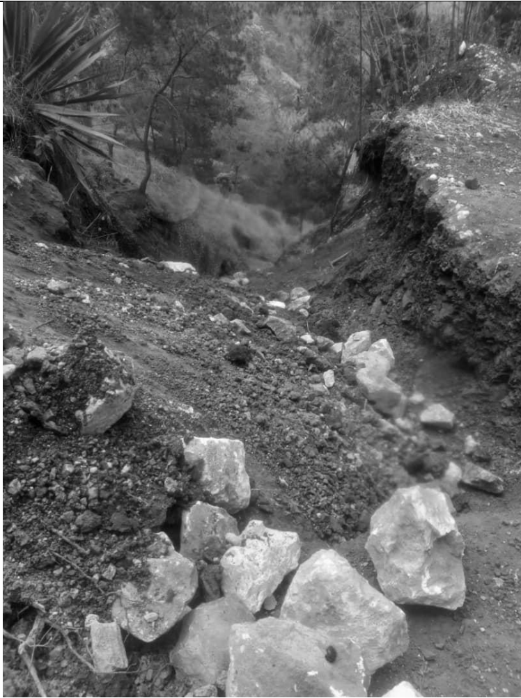
Photograph provided by local source in July 2025 showing parts of the road destroyed by gang
