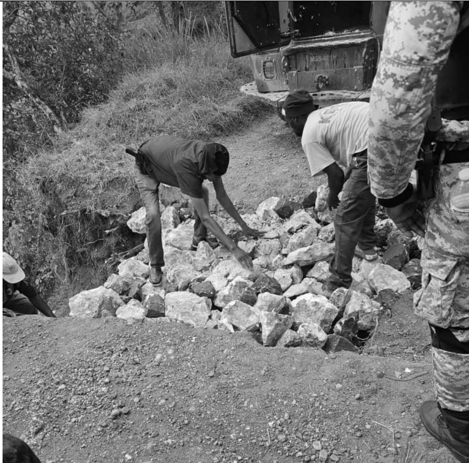
Photograph provided by local source in July 2025 showing police officers and residents filling in sections of the road damaged by gangs
