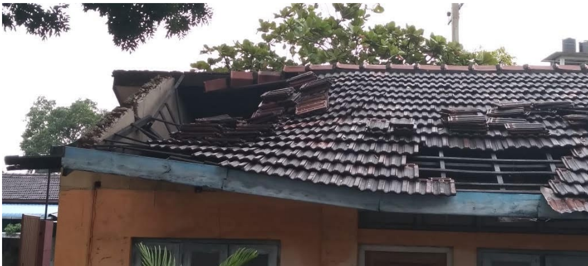
Damage to the roof of a school in Ampara, Sri Lanka. © 2025 Human Rights Watch
