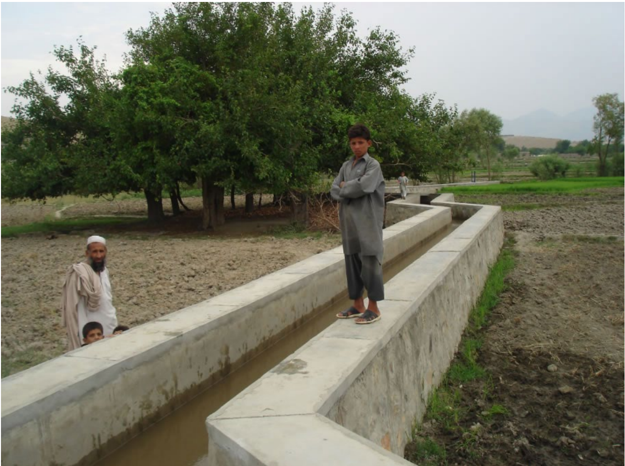
A micropower facility in Qarghayi district, Laghman province, which was built with support from the National Solidarity Programme (NSP).
