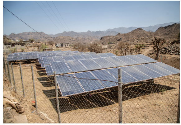
Solar panels provided by UNICEF to pump water from wells to houses in Al Odayn District in Ibb Governorate. © Ibrahim Almashriqi, UNICEF.
