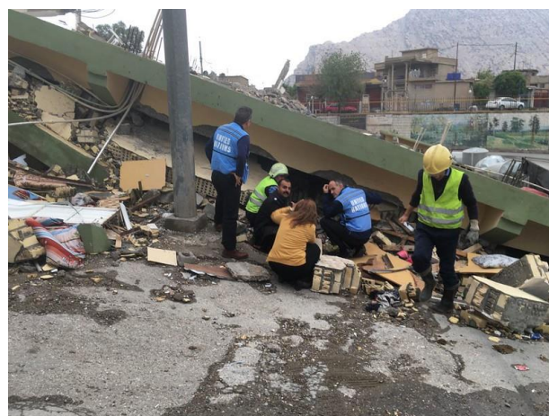
Civil Defence and UNDAC team inspect a collapsed building in Darbandikhan town. Photo Credit/UNDAC
