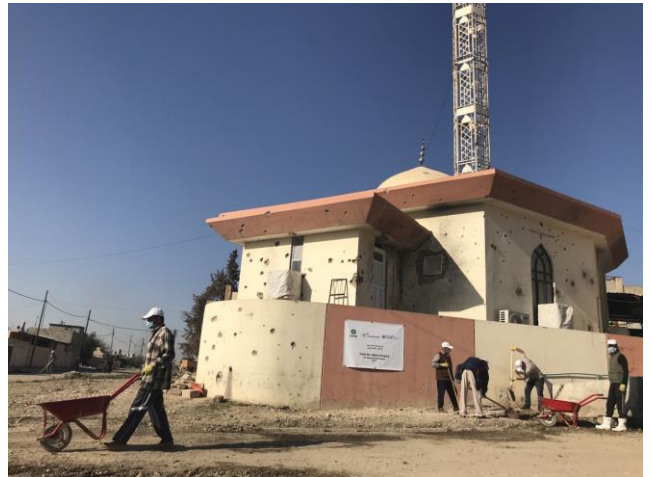
16 November 2017, Al-Mansour, west Mosul. Through the cash-for-work programme to rehabilitate the city's destroyed infrastructure, the IHF supports families affected by the conflict to rebuild their livelihoods and communities. Photo credit/OCHA
