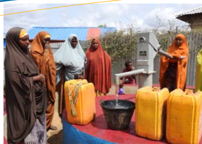
Rehabilitation of water points remains very critical ahead of the Deyr rainy season.
