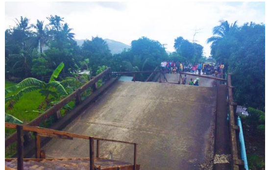
Credit: OCHA/M. Malang San Francisco, Surigao del Norte (14 February 2017) - The Anaon Bridge split into three places during the earthquake, cutting off access to Surigao City. Vehicles are crossing a river as a detour, which may be impassable during heavy rains.
