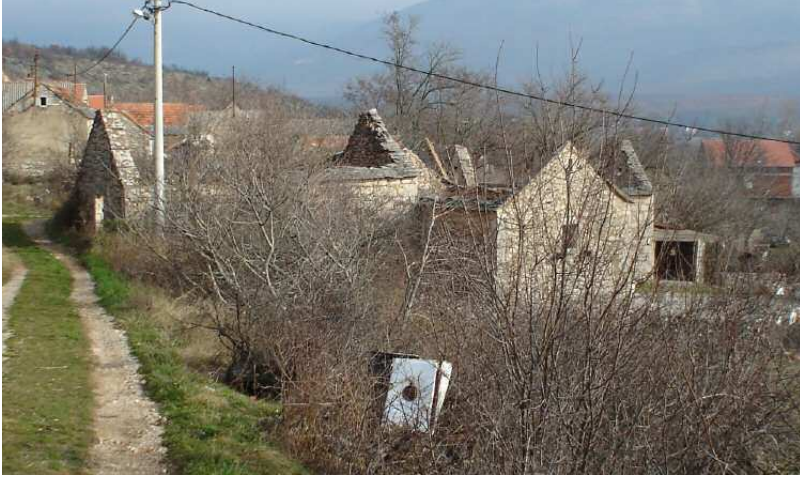
The slow pace of reconstruction of war-torn houses remained a serious obstacle to refugee return. Devastated houses in the village of Civljane. © CHC
