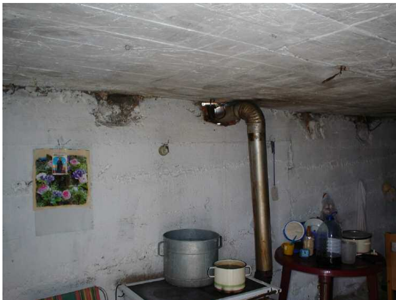
A returnee couple living in this one room of their house in the village of Cetina filed a request for reconstruction in 2001 and was still waiting for a decision in 2006. The roof leaked and the room had no heating. © CHC
