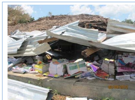
Photo 2: Damaged TLS in Zone 1. Credit: UNICEF
