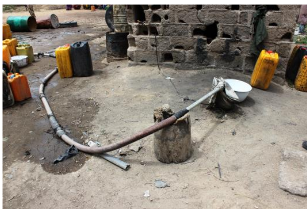
Water pump and generator at one of the five water points.
