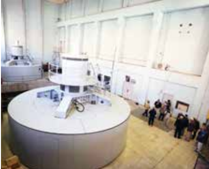
U.S. officials view the dynamo room at the Kajaki Dam. (U.S. State Department photo by Musadeq Sadeq)
